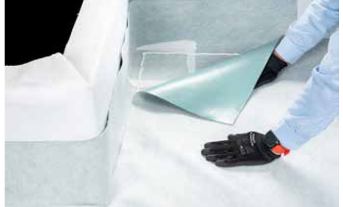
The corners and angle areas are sealed using pieces of membrane RENOLIT ALKORPRO shaped and sealed with the RENOLIT CEM 805 mastic glue.
