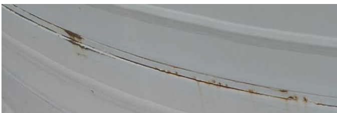
Visible signs of corrosion around a flange
