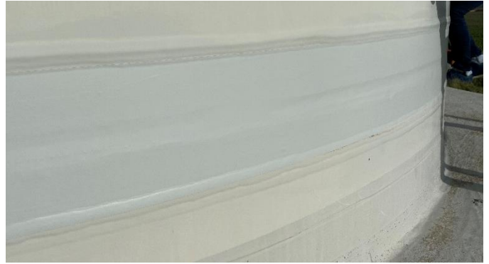
This shows the standard RAL colour “light grey” of the RENOLIT CP compared to the faded original paint finish which was originally the same colour.
